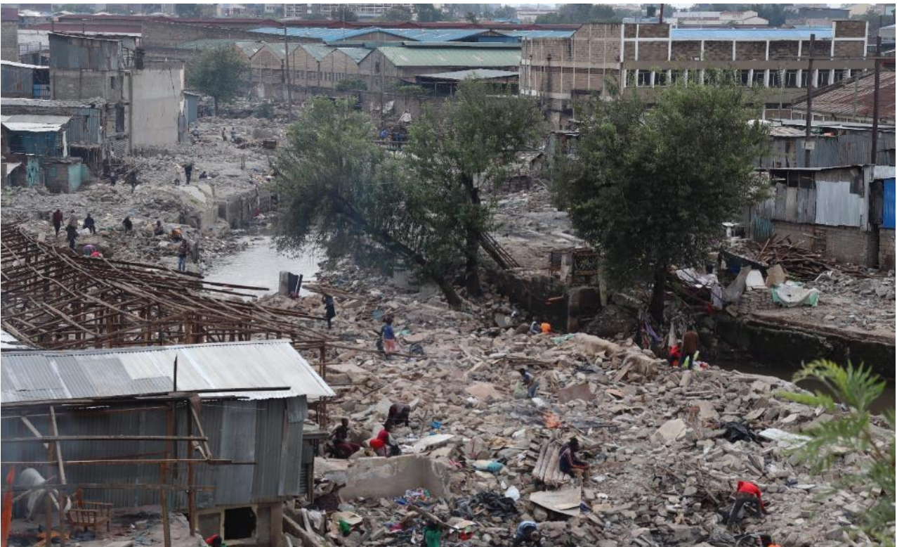
Hundreds of homes destroyed by the demolition in Mukuru Kayaaba
