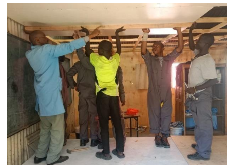
Charles and the carpentry boys are renovating the old mabati classroom into a gallery and exhibition room.
