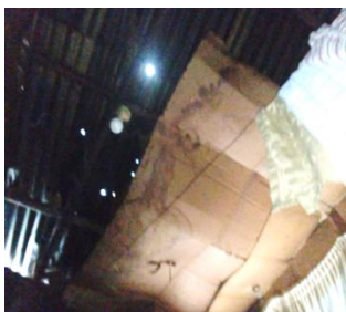
Roof was destroyed
